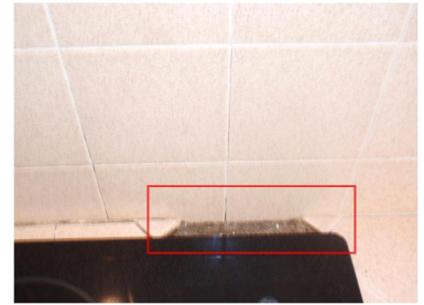
Missing tile at stove top
